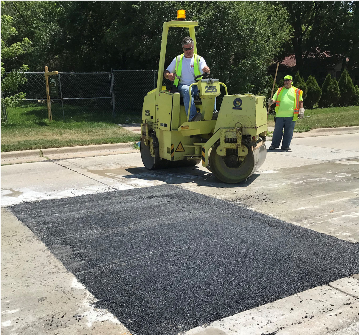
Cook County maintenance crews repair and maintain asphalt and concrete pavement surfaces, ensuring safe and efficient traffic flow on Cook County roadways.
