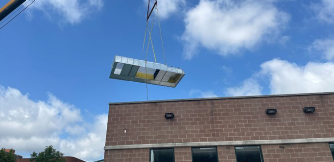
Installation of new roof top air handling unit at Provident Renal Dialysis Clinic
