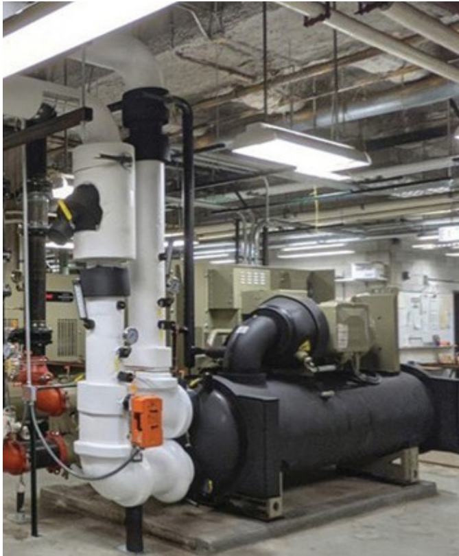
New Energy Efficient Chillers at the Institute of Forensic Medicine
